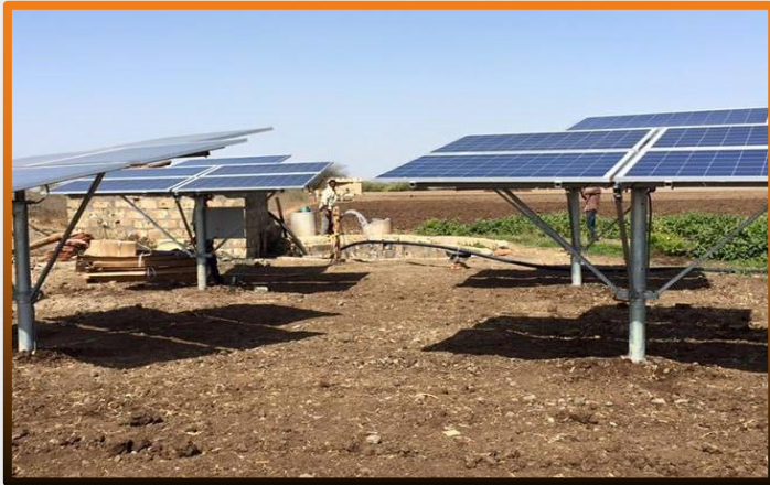
Solar Water Pumping Projects
