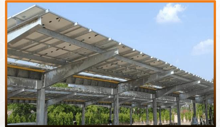
Solar Car Port Projects
