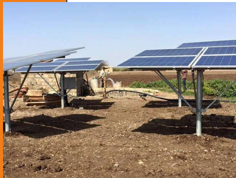
Solar Water Pumping Projects
