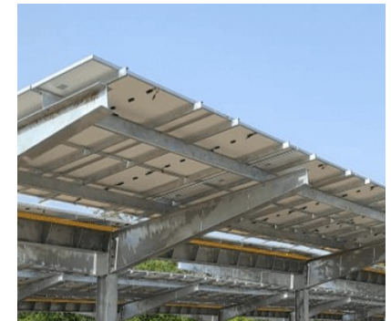
Solar Car Port Projects
