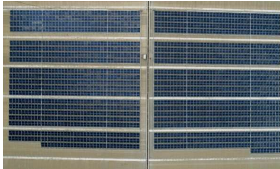
Industrial Solar Rooftop Projects
